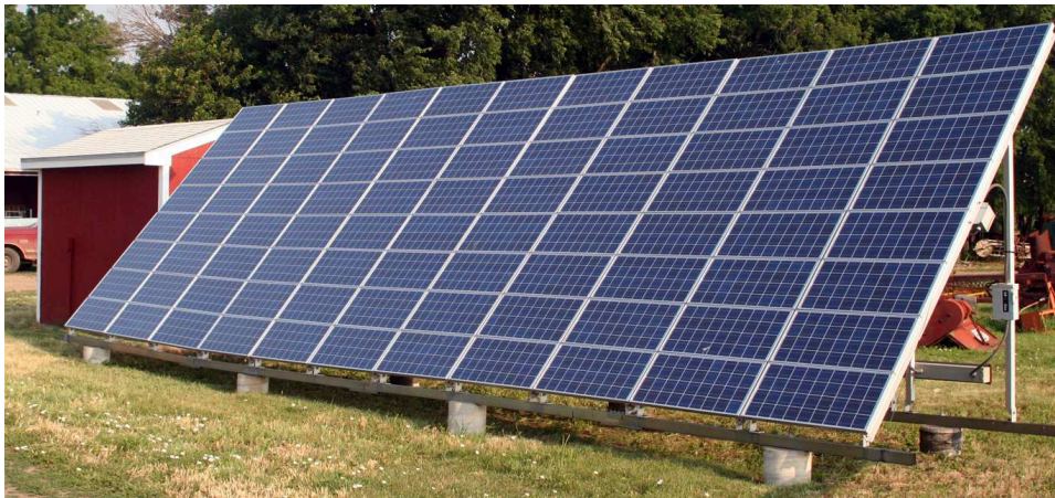
Figure 10: The Sunshine Farm solar array, with battery-storage and electronics shed.
